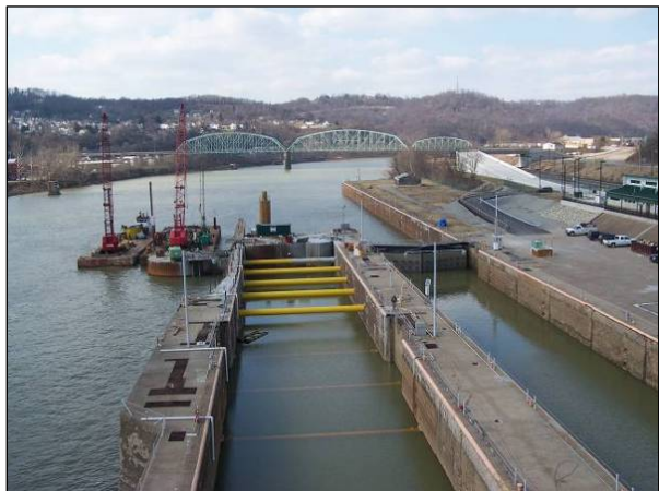
Construction of the stabilizing struts and downstream closure as part of the River Chamber Demolition contract.
