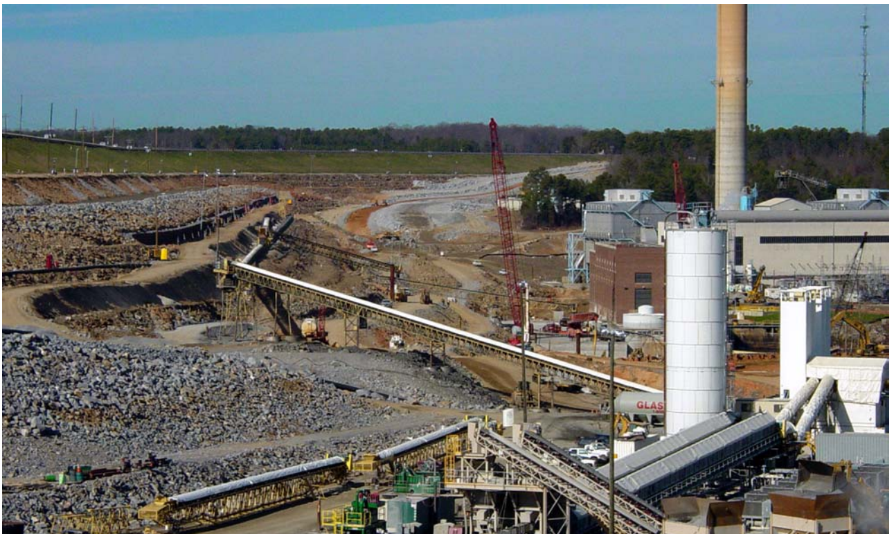
Figure 2 RCC Batch Plant and Conveyor
