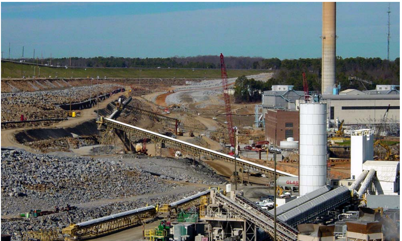
Figure 2 RCC Batch Plant and Conveyor
